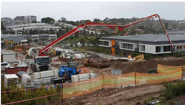
Figure 15: Concrete boom-pump operation requires approval when operating on and/or above a road.
