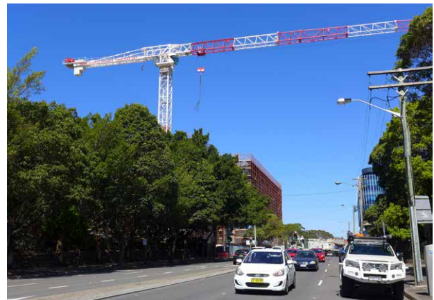
Figure 12: Approval under the Roads Act is required when any part of a hoisting device swings or operates over a road including under wind-vaning actions.
