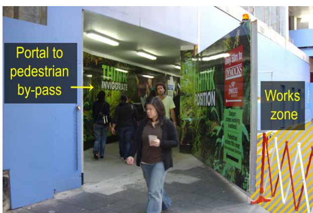
Figure 40: The hatched area indicates a works zone on a temporarily closed footway (operational only during approved works zone times) with a pedestrian by-pass through a fully enclosed protective tunnel within a construction site.
