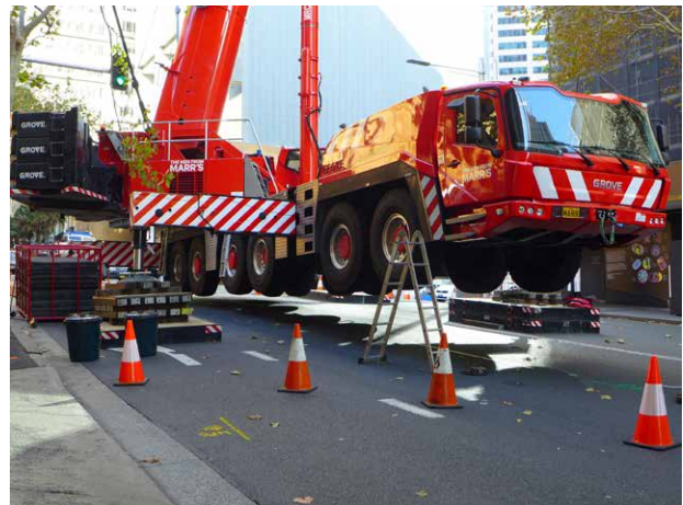
Figure 2: Bearing pressures transferred through outriggers must be evenly distributed to prevent damage to roadways . Outriggers and crane bodies must not encroach on through-traffic lanes.
