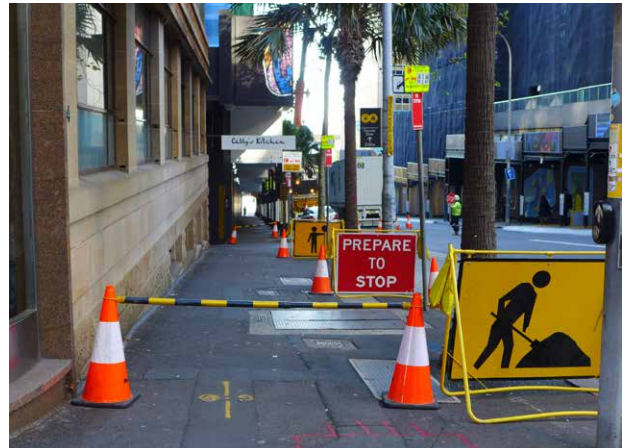
Figure 4: Required signage in accordance with AS 1742.3 and the TMP must be displayed clearly.
