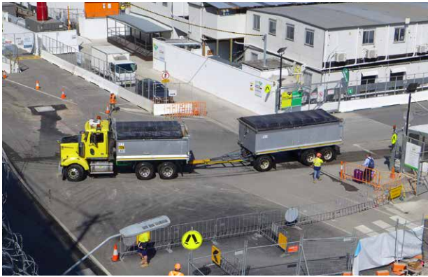
Figure 23: Loads containing demolition material, soil, sand or excavated material must be fully covered before entering the road network.
