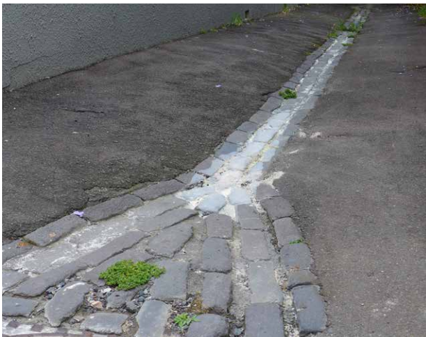
Figure 47: Cobble stormwater drainage gutters and stone kerbing are important historic fabric of the City and must not be damaged or removed when undertaking works within public places .
