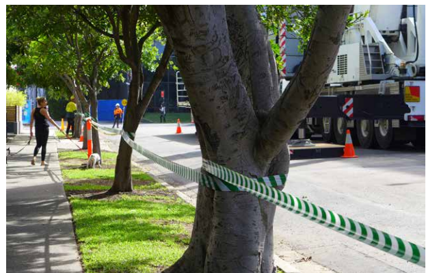
Figure 7: Appropriate barriers must be installed to isolate an approved work / crane operation area . In busy pedestrian areas such as the city-centre , metal barriers must be used.
