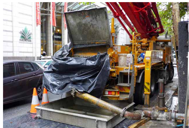
Figure 18: Pollution prevention measures must be in place during concrete pumping operations to prevent spillage onto roadway surfaces and pollution offences (stormwater pollution).
