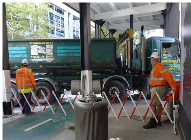
Figure 41: The control and safety of pedestrians and bicycle riders at truck access points is essential. This is particularly important in high volume pedestrian areas. The City will allow, and require, the use of manned concertina gates as a control measure .
