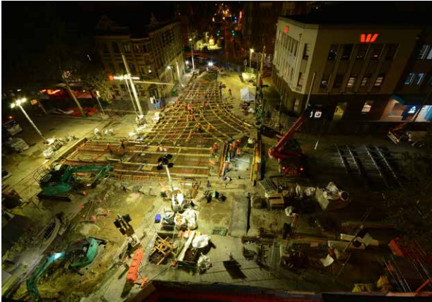
Figure 37: The use of temporary lighting systems must avoid loss of amenity within the local neighbourhood through selecting and positioning lighting systems that prevent light-spill and glare. (Image courtesy of Transport for NSW)
