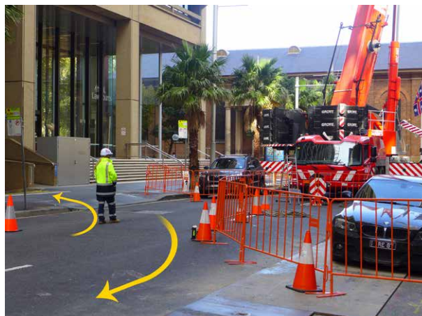
Figure 21: Unless otherwise specifically permitted, access to buildings including vehicle access must be maintained during temporary road closures.
