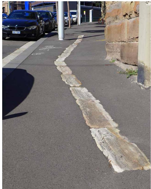
Figure 48: Significant sandstone kerb stones marking the original location of the roadway / footway alignment. Such features must not be altered or disturbed without first obtaining the approval of the City .
