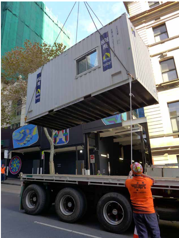
Figure 11: All hoisting operations must be carried out within the confines of a works zone or a temporarily closed traffic lane (to a height of at least 4.5 metres above the road surface).
