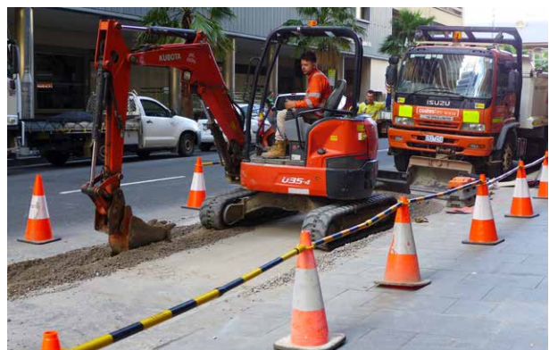
Figure 28: Road opening works must be isolated from the public accessible space by barriers as determined by the PCBU or the City (where directed or required).
