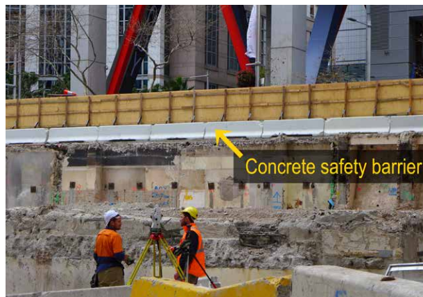
Figure 44: Excavations (deeper than 1.5 metres) must be protected by suitable barriers that the PCBU determines is required and is of an acceptable design to withstand all likely impacts including vehicular impacts.
