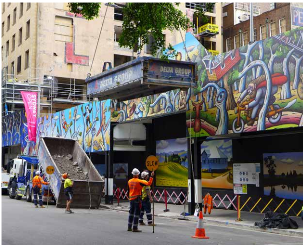
Figure 34: Through-traffic must not be stopped during hoisting operations from a road . For wide loads (greater than 2.4 metres) traffic can be temporarily stopped for a short duration until the load has reached a height of 4.5 metres above the roadway (subject to meeting prescribed requirements).
